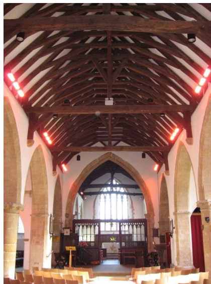
Photo: The new nave heaters in place, February 2019; Tony Hughes
