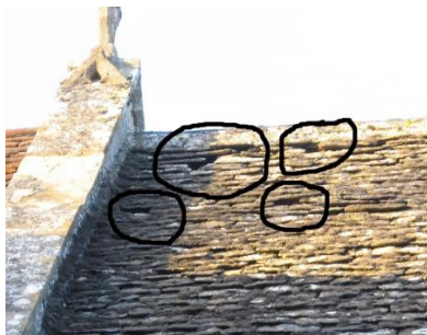
Photo: Missing stone tiles on the chancel roof, November 2021; Tony Hughes
