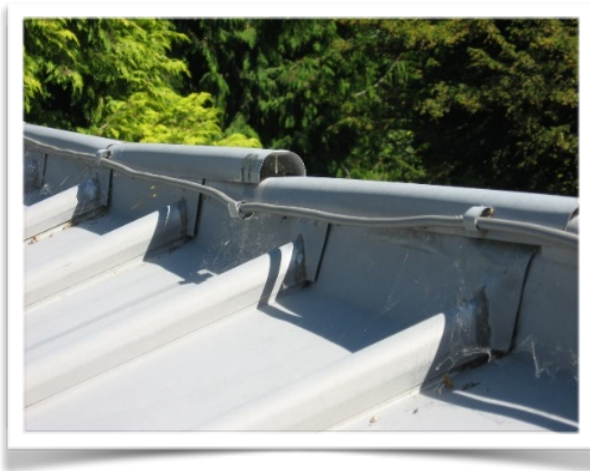
Photo: Lifted ridge of extension roof, August 2022: Tony Hughes
