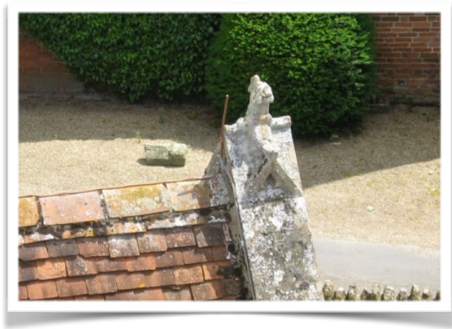
Photo: Remains of finial cross on South Transept roof; Tony Hughes
